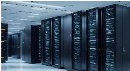
Data Center Cooling
